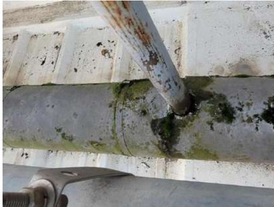
Figure 7. Algae on the ammonia pipe jacketing.
