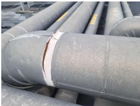
Figure 3. Jacketing separation and split seam
