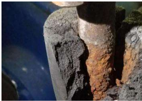
Figure 6. Elastomeric foam insulation on ammonia piping.
