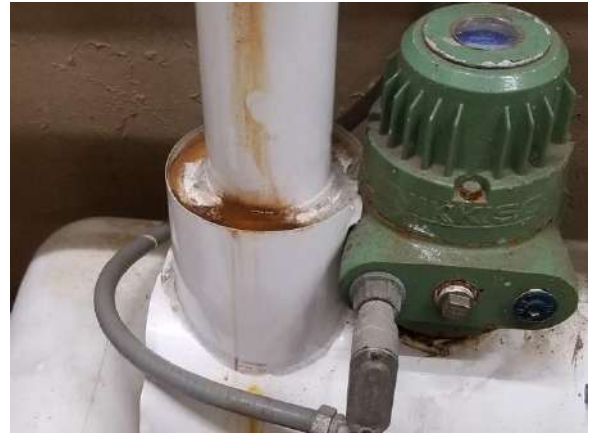
Figure 5. Water pooling at the base of insulated ammonia piping at pump out.
