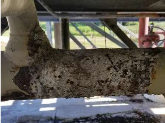
Figure 4. Chemically induced corrosion on bare piping.
