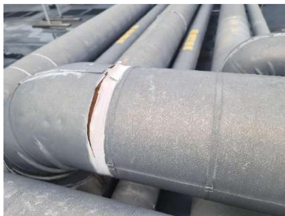
Figure 3. Jacketing separation and split seam
