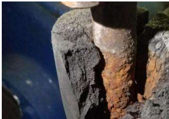
Figure 6. Elastomeric foam insulation on ammonia piping.
