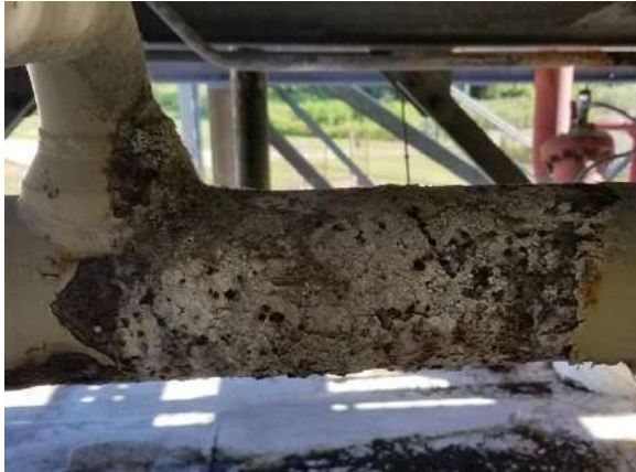
Figure 4. Chemically induced corrosion on bare piping.
