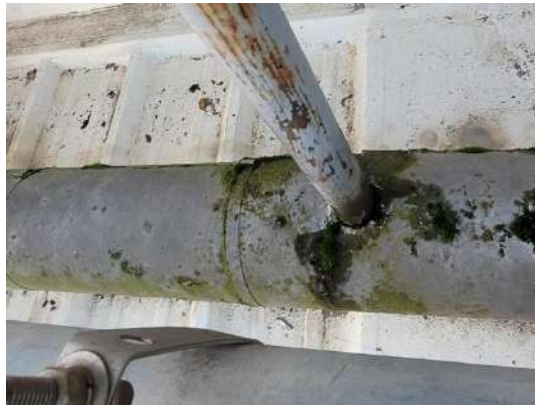
Figure 7. Algae on the ammonia pipe jacketing.
