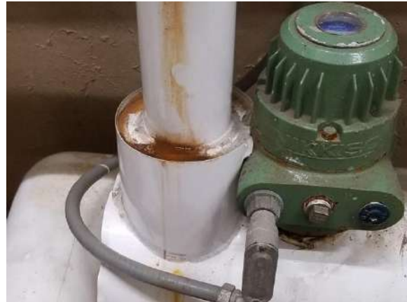
Figure 5. Water pooling at the base of insulated ammonia piping at pump out.
