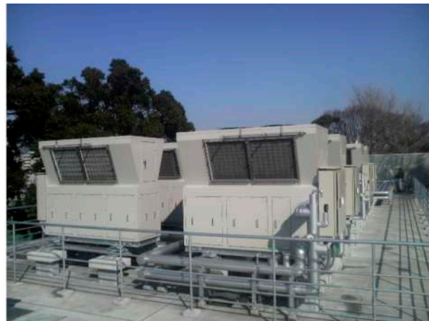
Fig. 14 New chillers with hermetic ammonia scroll and conventional condensers
