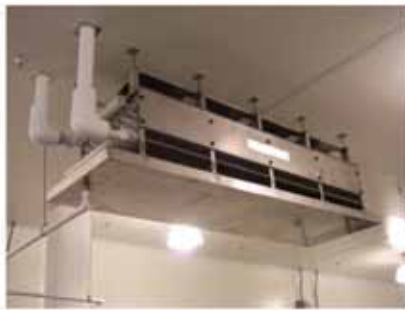
Ceiling suspended air cooler
