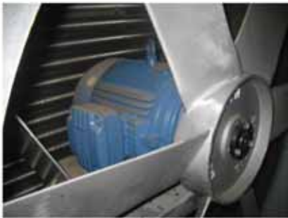
Typical air cooler axial fan assembly
