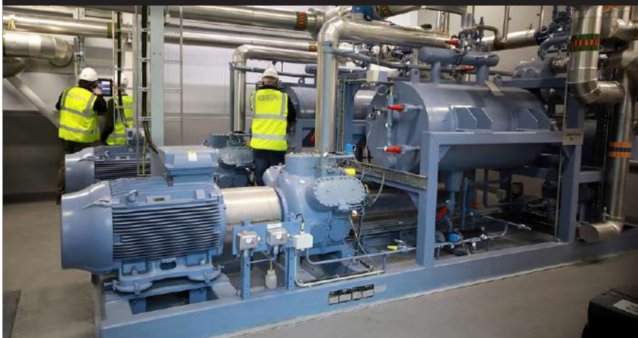
Figure 5. Installation of 1,200 kW ammonia heat pump at Aurivo fresh milk dairy in Ireland.
