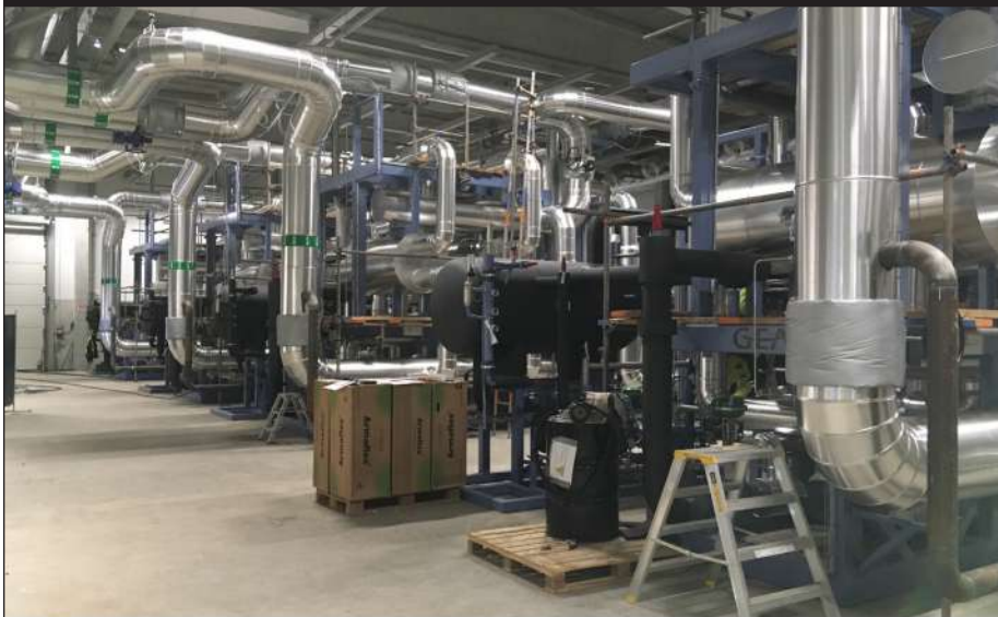
Figure 9. Four 10 MW heat pumps installed in Malmö, Sweden.
