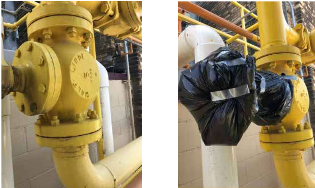
Figure 2. Shutoff valve on the high-pressure side of an ammonia refrigeration system (left) being bagged (right) to quantify refrigerant leakage from the bonnet gasket or stem packing.
