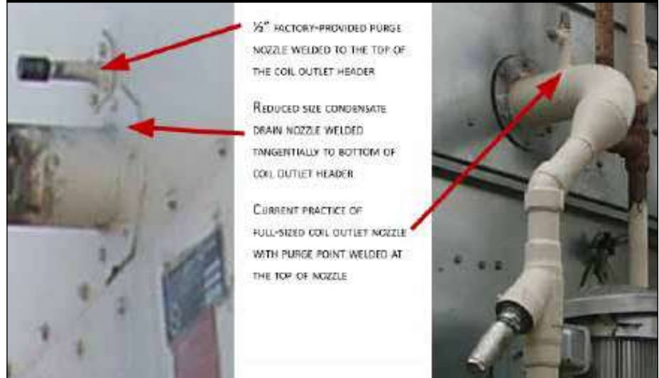
Figure 2. Former construction method of the purge point installed by the factory, and the current practice of field-installed purge point.
