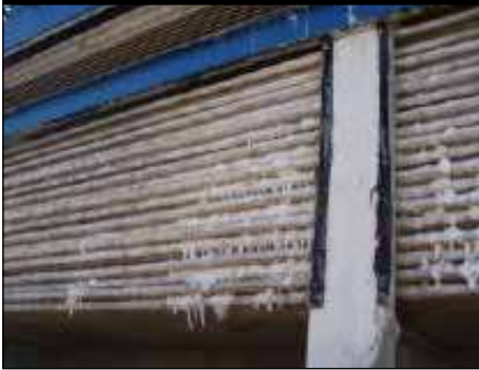
Figure 1. Consequences of poor condenser operation.
