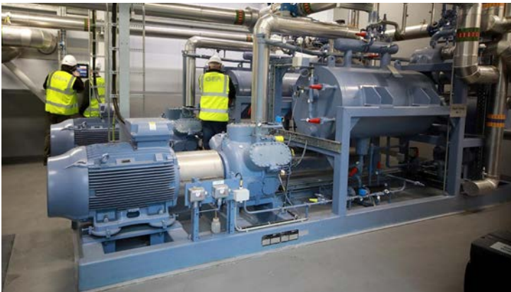
Installation of 1,200 kW ammonia heat pump at Aurivo fresh milk dairy in Ireland.
