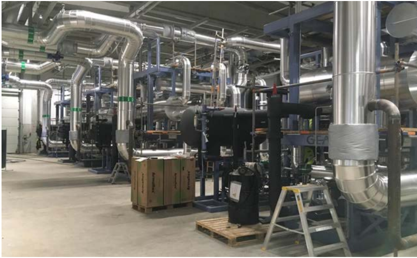
Four 10 MW heat pumps installed in Malmö, Sweden.
